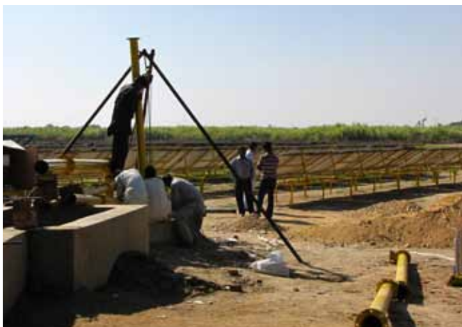
Figure 12: Solar energy fuelled pump.
