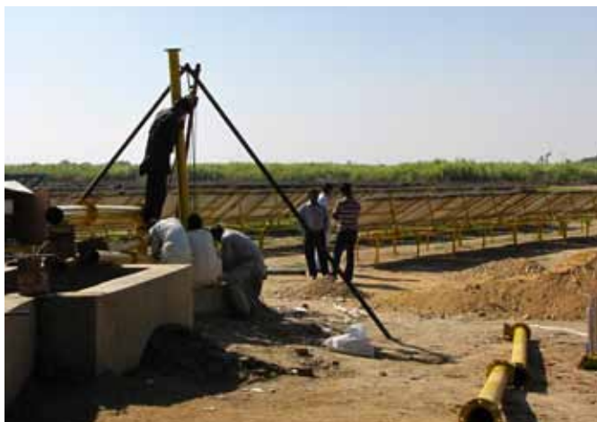
Figure 12: Solar energy fuelled pump.
